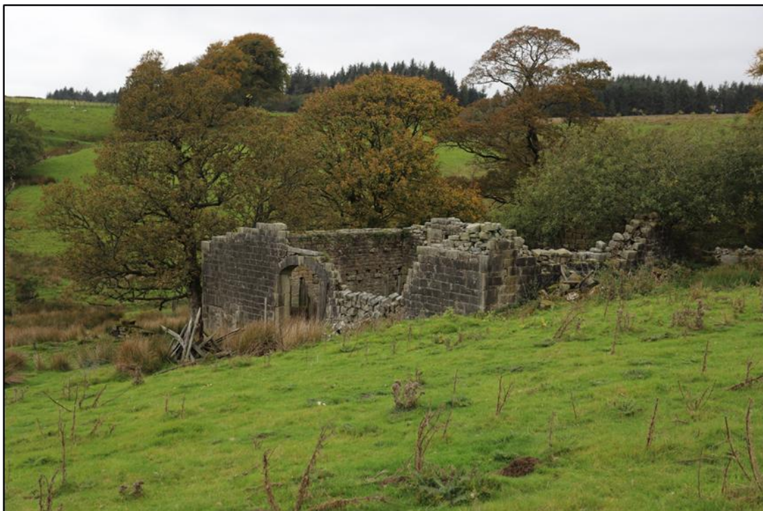
Photo 7: Derelict building illustrated as “Lower Lathe” on the 1851 OS Map looking northwest
